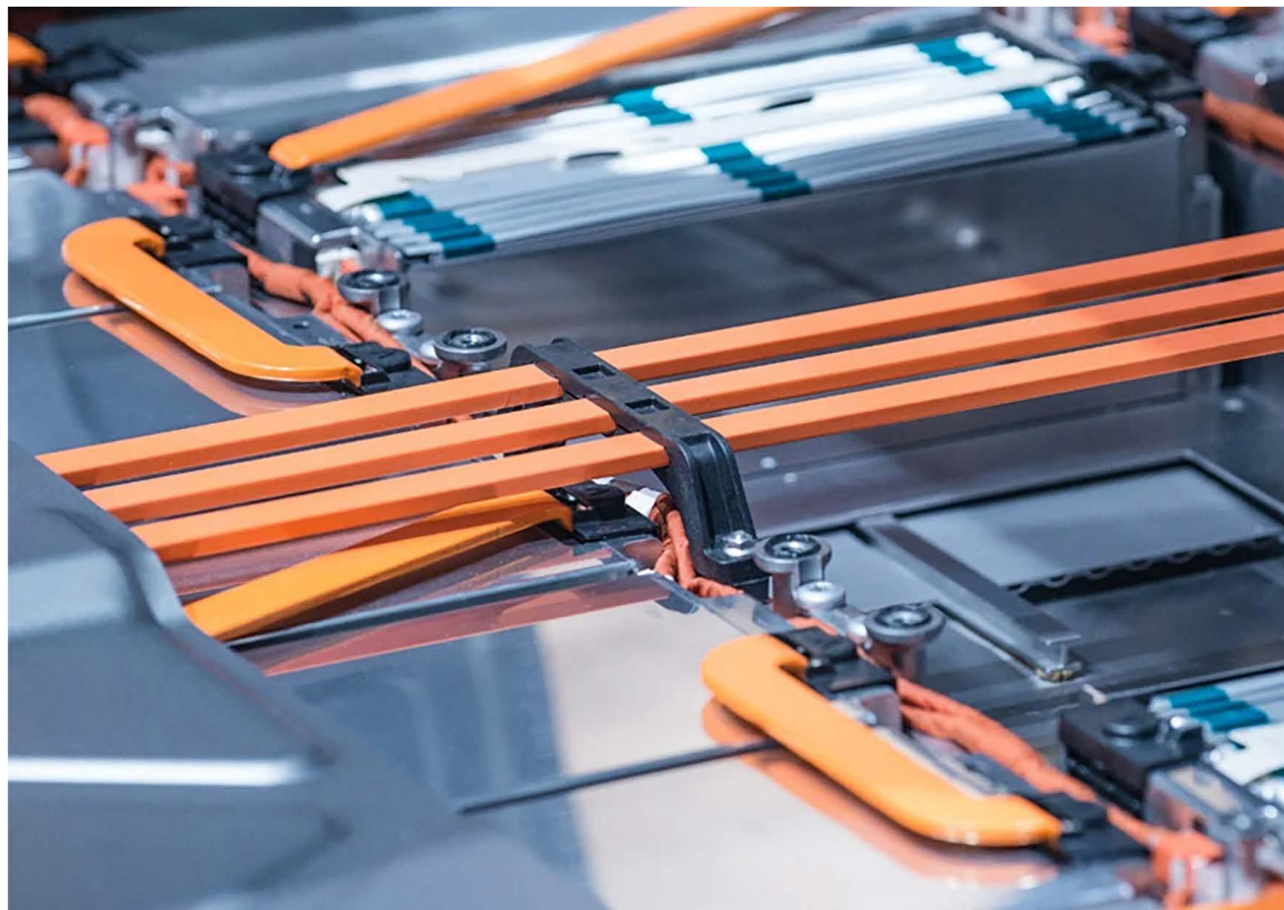
Fig. 3 Busbars inside the battery compartment of an electric vehicle
