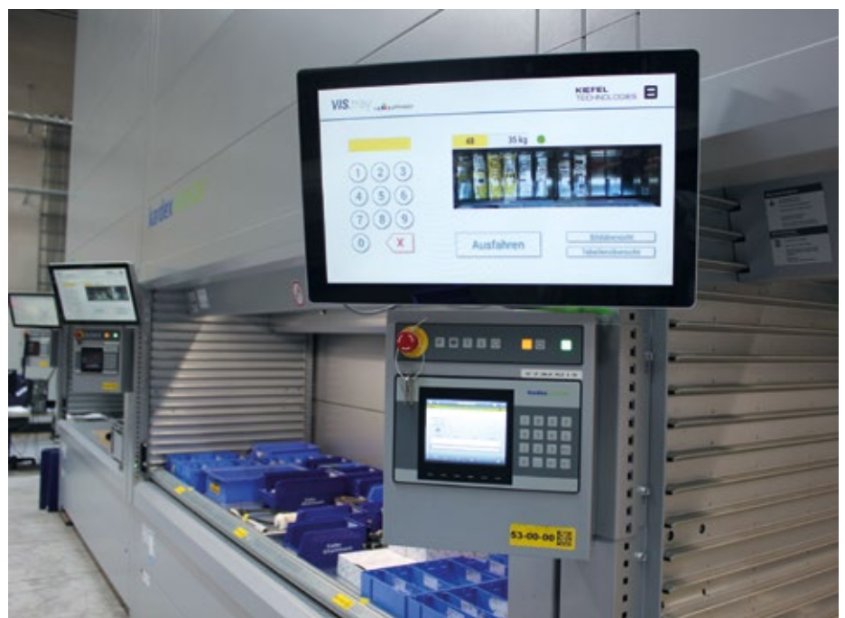
The installation requires communication between the Kardex high rack controller (below) and the image capture system.
