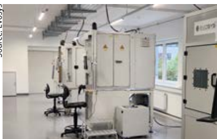
Production area in the new ELS building in Erlangen, Germany (Source: Evosys)
