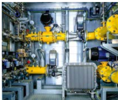
The spectrometer and the hydrogen sensor installed on a natural gas bypass. (Source: Fh.-IPM)
